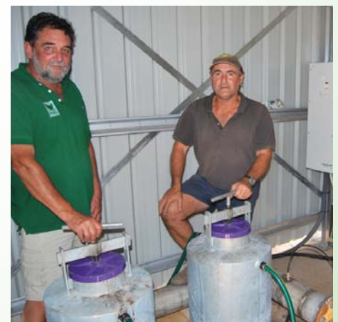
Peter and Lou with the Curino’s new pump system that has allowed them to dramatically lower pressures and cut their electricity bill in half.
