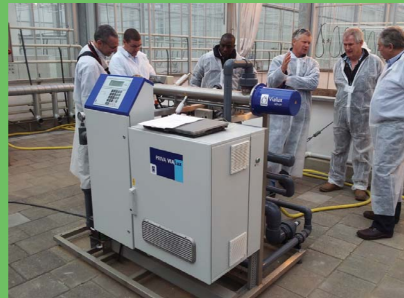
Water treatment systems using both ultra violet and hydrogen peroxide are being evaluated for water sterilising efficacy.
